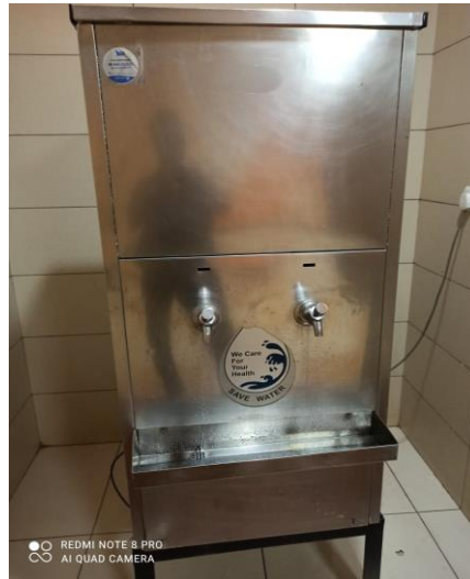
RO WATER COOLER
